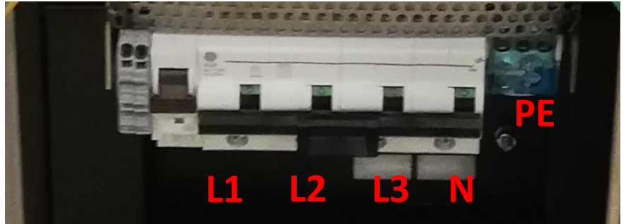
Figure 17: Connection of charging station to the power grid
